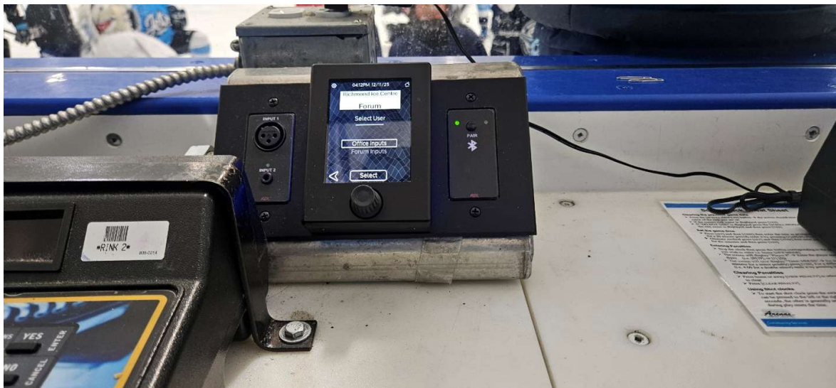
RDL-VR2-RDL in custom-made pod, all PoE powered with 5-port switch
