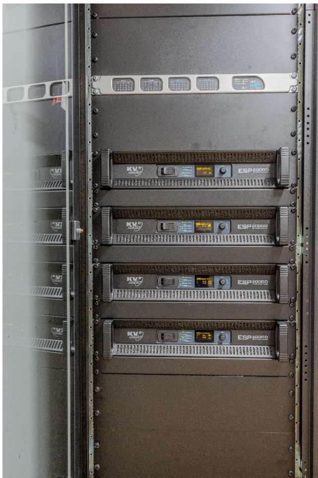
First of two amp and processing racks, VMX88 at the top
