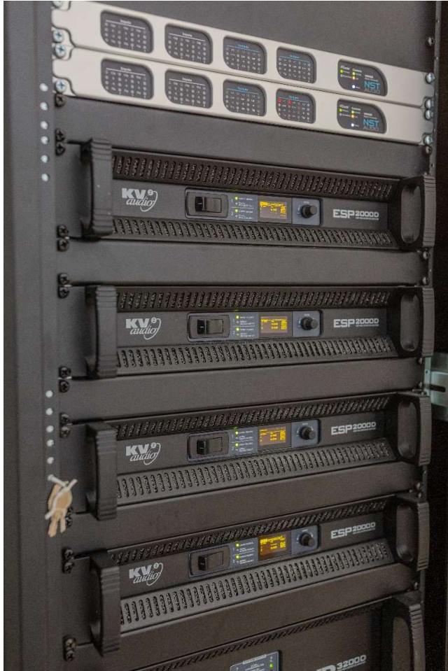
Second rack with a pair of VMX88s in control
